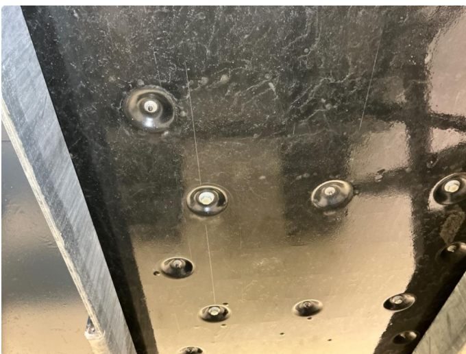
2.1 Riper i plate under batteri - ok
