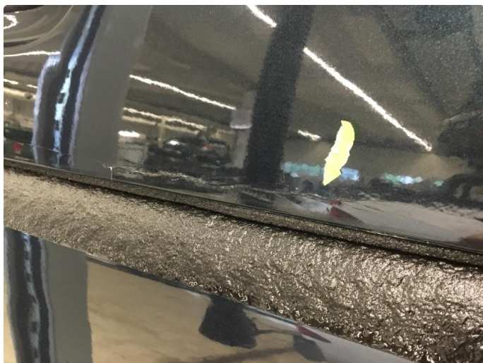
1.1 Sprekk i gailcoat h.side plantopp.
