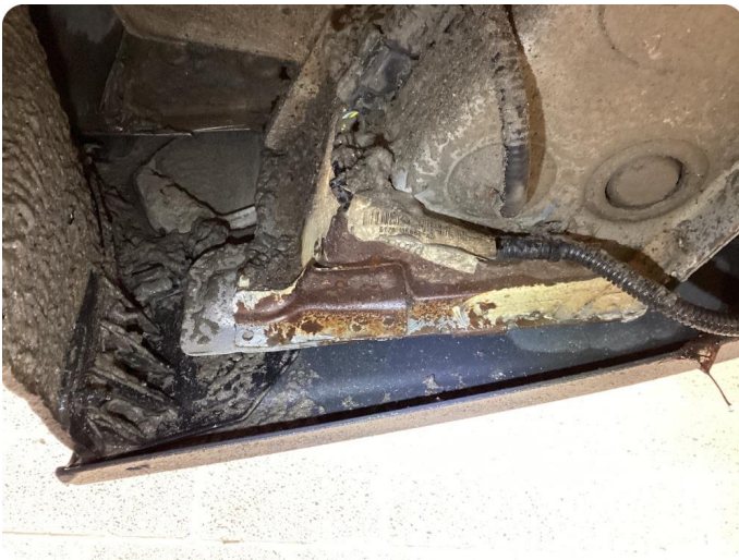
1.2 Rust Anbefaler rust behandling under
